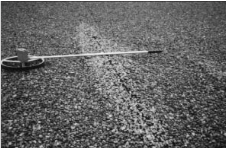
Figure 1. Blistering occurs when pockets of air and moisture trapped between the plies of the membrane, or between the membrane and substrate, expand and displace the membrane.
