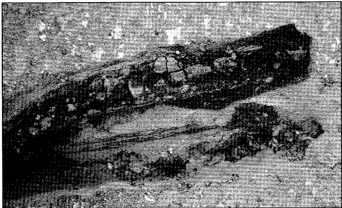
Figure 16. After micro-cracks have appeared at the aggregate-bituminous binder interface, aggregates can be pulled out of their bed by a strongly adhering sealant.
