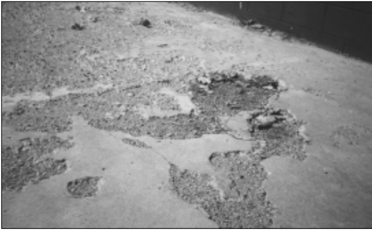
Figure 2. Deterioration of concrete deck
