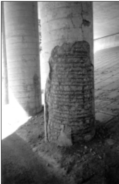
Figure 1. Deterioration of bridge pier due to de-icing salts from wheel spray
