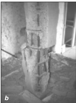
Figure 1. View of (a) normal-strength concrete column and (b) high-strength concrete column after fire-resistance tests
