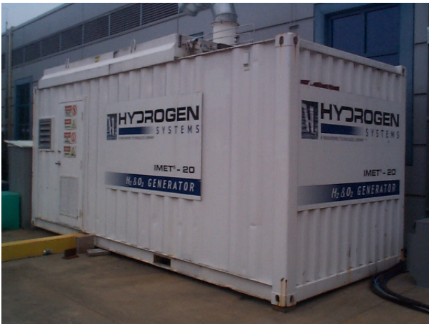
Figure 2: IMET-20 Electrolyzer at NRC
